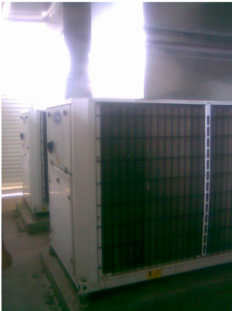
Fig. 1 Carrier chillers located in a north-west compound with corrugated walls and roof that is heated up by afternoon sun
