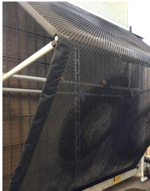
Fig 2 Carrier chiller 1 with a 1.2 m EcoMesh and dual sprayers installed
