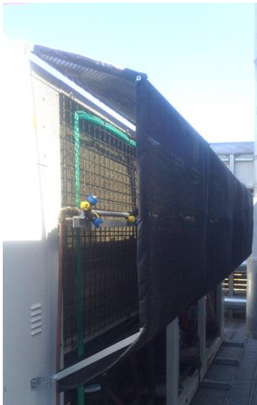
Fig. 1 EcoMesh (4 panels) mounted along the front of the chiller
