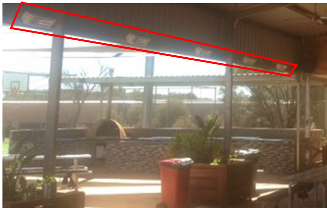
Now overhead electric heaters warm people in the courtyard, eliminating the need for cumbersome gas patio heaters.
