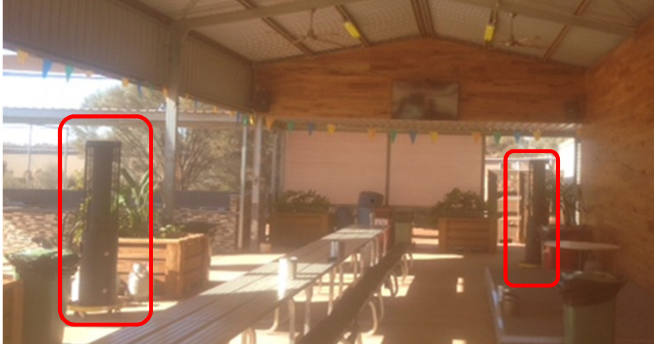
Typical mine camp courtyard area with gas patio heaters.
