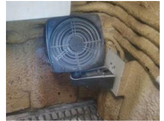
A common solution for keeping equipment warm in a lubrication container - a residential fan heater
